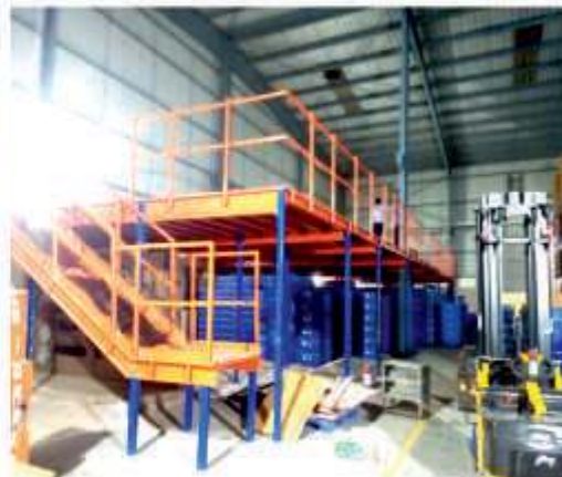
Modular Mezzanine Floor
