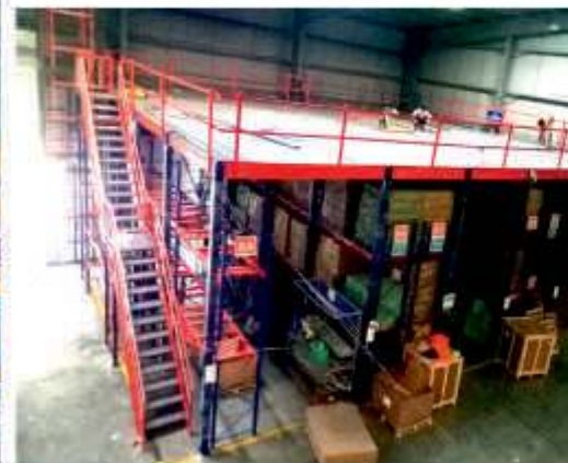
Modular Mezzanine Floor
